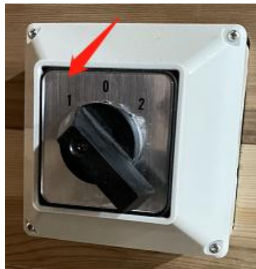
Power to stove heater
